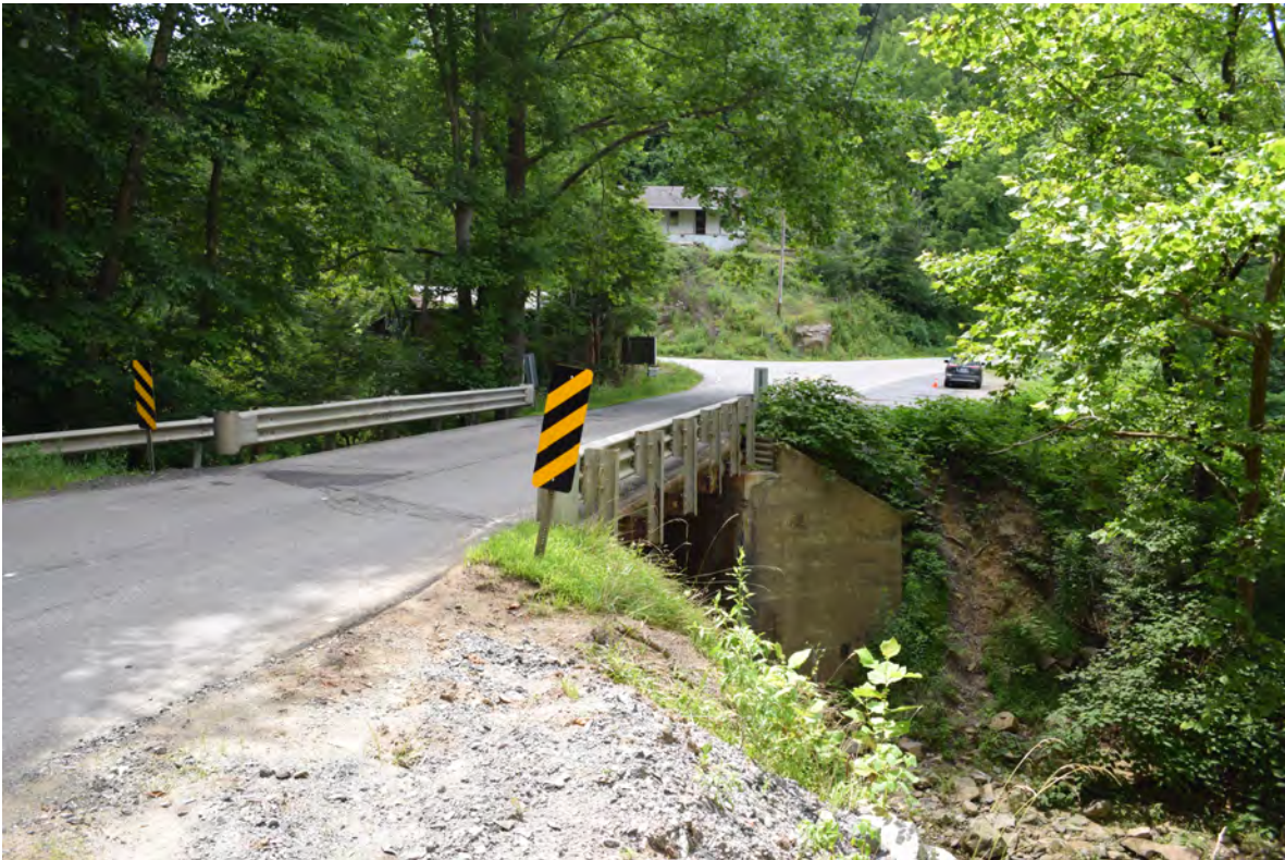
Bridge No. 84 on NC 209, view to the northwest with the Jack Caldwell House (MD0300) in the background
